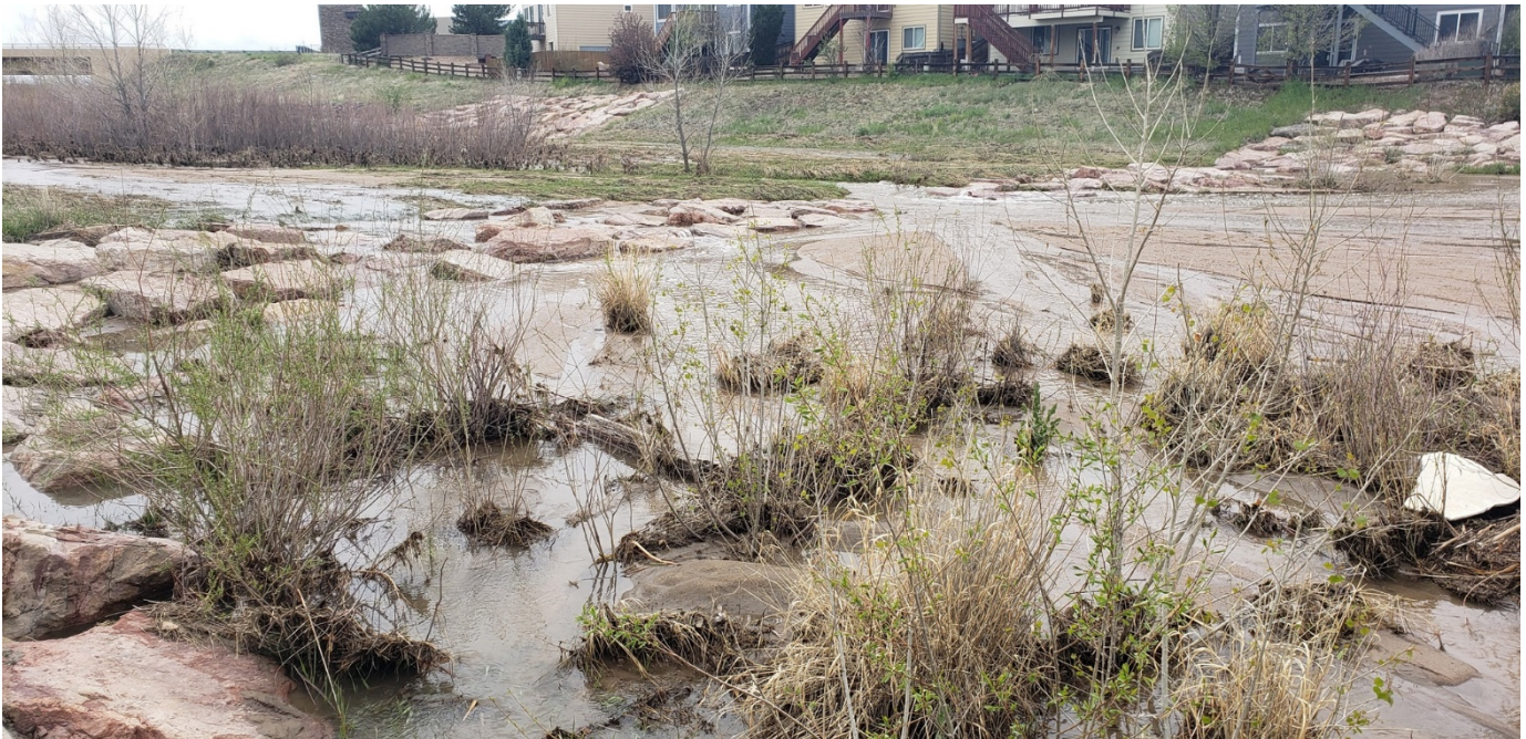
Figure 1: Photo Downstream of Jordan Road at Drop Structure (Photo courtesy of SEMSWA, 2023)
