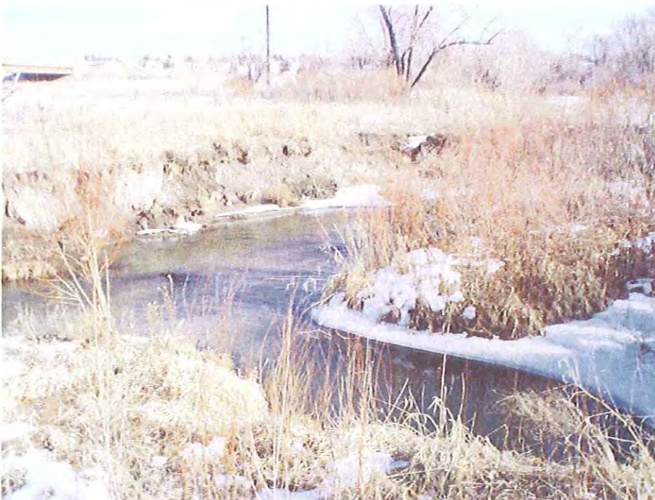
PHOTO 2 – CHERRY CREEK BANK EROSION AT CONFLUENCE WITH HAPPY CANYON CREEK
