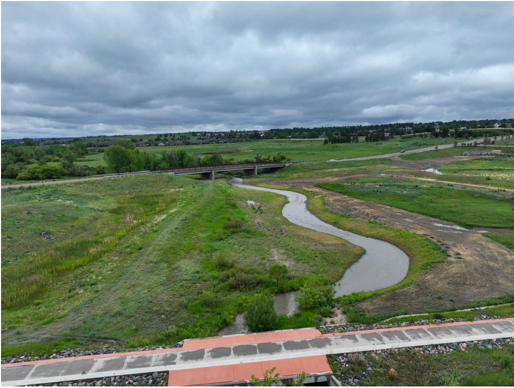
Figure 8: Cherry Creek at Downstream Limits of Project (Courtesy of Naranjo Civil Constructors)
