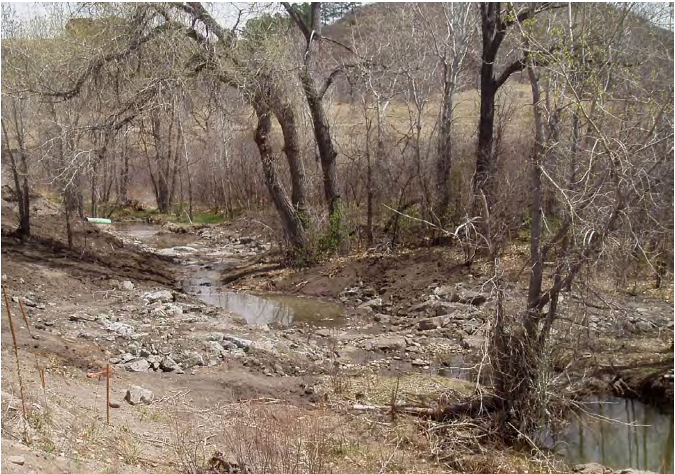
Boulder cascade drops being constructed at critical locations to protect the Gulch against major erosion while preserving existing riparian vegetation.
