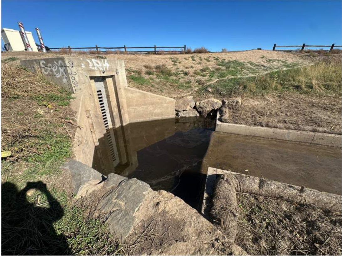
Figure 3: Pond W6/7 –Outlet Structure with Concrete Micropool
