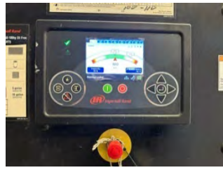
Compressor running normally
