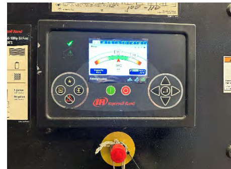
Compressor running at normal operating pressure
