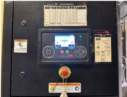
Compressor running normally at 100 psi
