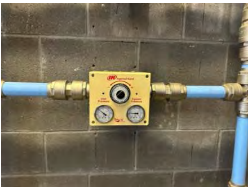
Compressor restarted and running at 55 psi
