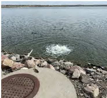
Leak detected near distribution manholes
