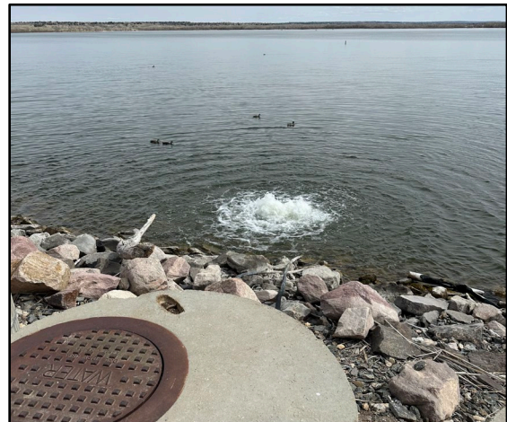
Broken main air distribution line near the distribution manifold
