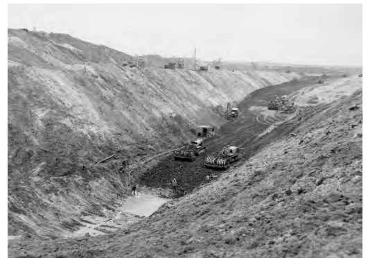
CHERRY CREEK DAM - 4 April 1947 Looking toward left abutment at equipment placing backfill in cutoff trench.
