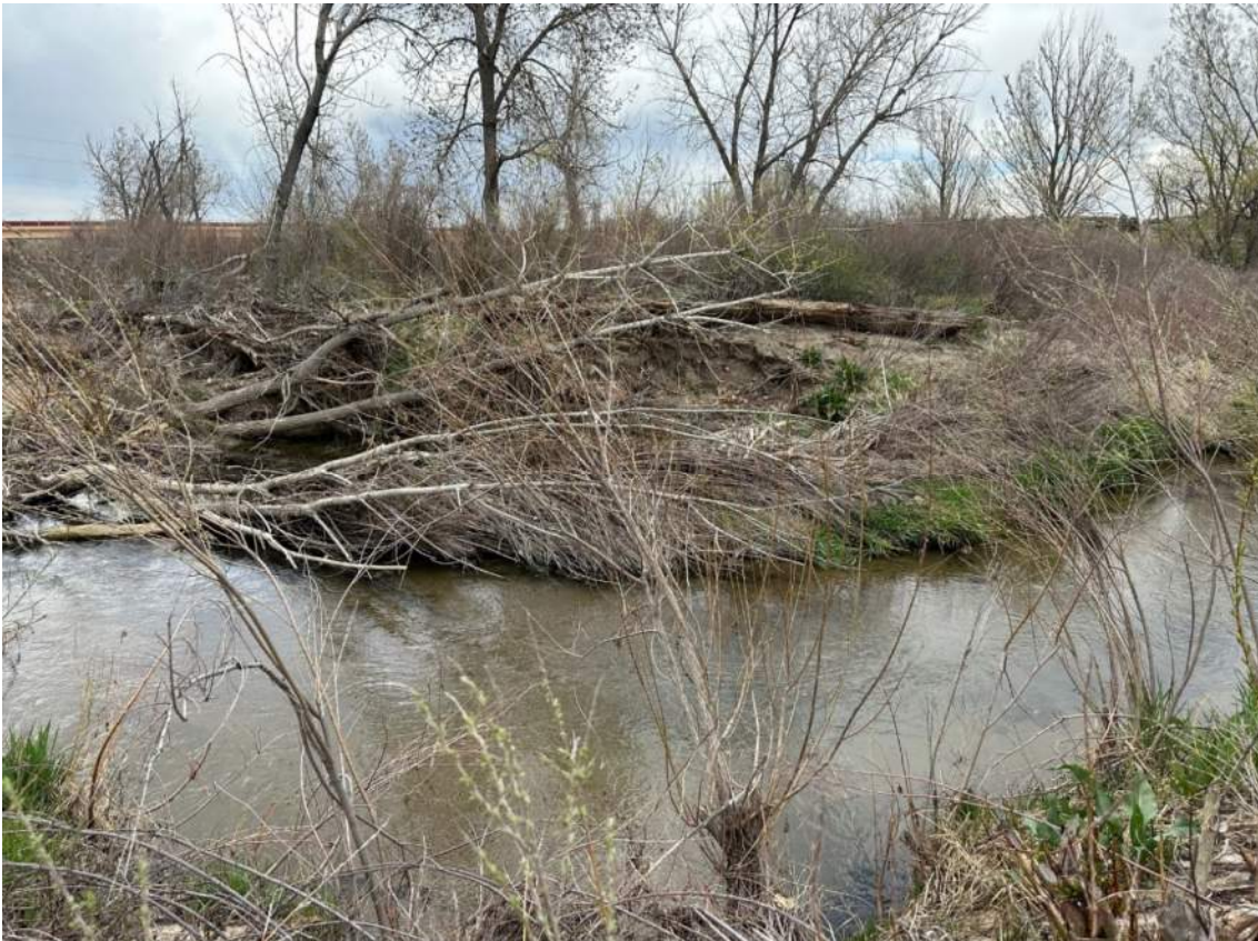
Figure 1: Bank Erosion Upstream of Arapahoe Road
