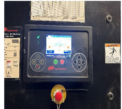
Normal compressor operating pressure
