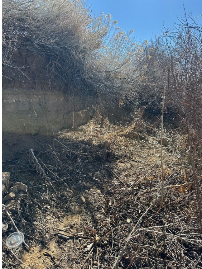
Figure 4: Vertical Cut Bank (South Project Area)
